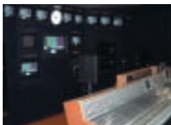
Editing equipment: Cameras and microphones are switched, and digital material, such as pictures and credits, stored on servers is input to assemble programs.
